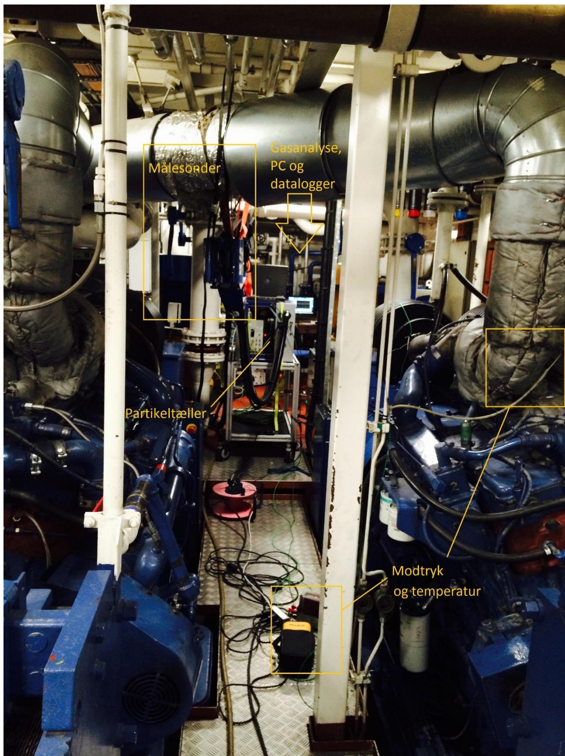
Figure 1: Test equipment (before mounting of filter). At the right you see the generator DG3, on which we perform measurements. In the background you see particulate counter, test probes and heated lines, which are mounted in the exhaust manifold above the passage. The back pressure transmitter is placed next to the engine connected to the outlet on the first bending after the turbo. At the front of the engine room the gas analysis instruments and the gas cooler are placed.
